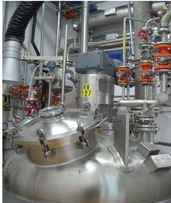
Hastelloy™ Cryogenic Reactor
